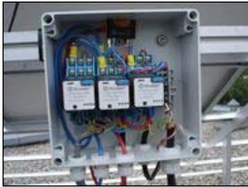
Figure 3: Switch box: multiplexing of 39 modules one shortcut relay, two change circuit relays each (FINDER 62.33.9.024.4040), current sensor (Isabellenhuette/Bader BMN4P/10H R010 0.1%) used for normal operation monitoring
