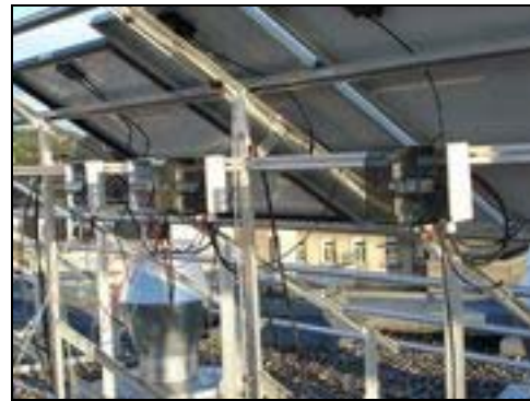
Figure 6: Connection of the switchboxes behind each PV module
